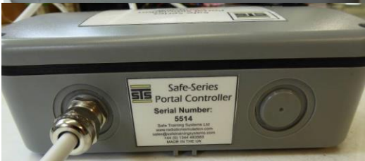
Cable to Portal Detector
